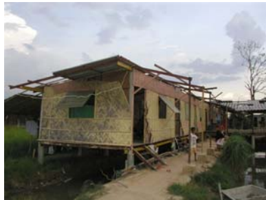
The shelter was destroyed beyond repair
